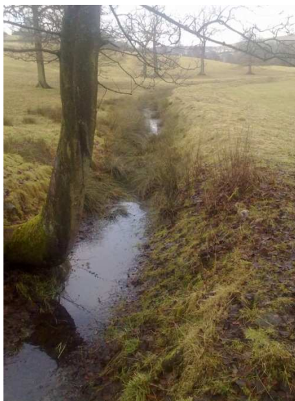
Figure 5 The leat from the intake weir to the mill is silted up
