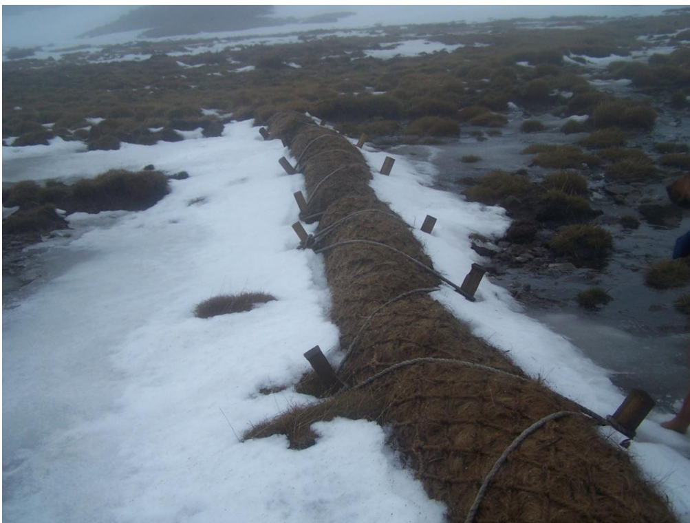
Example of coir log in situ on mineral soil at Holme House(from 2012 work), 14 Feb 2013
