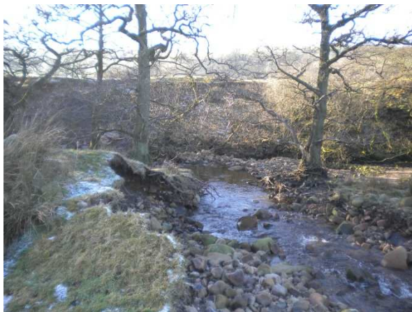
Figure 2 The position of the weir, now washed away
