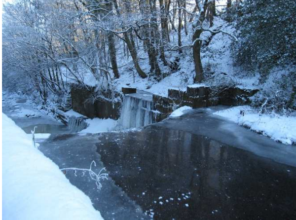
Figure 2 The weir from above with the old sluice gate on the far right and overspill
