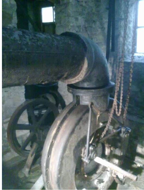
Figure 3 The existing turbine (damaged)
